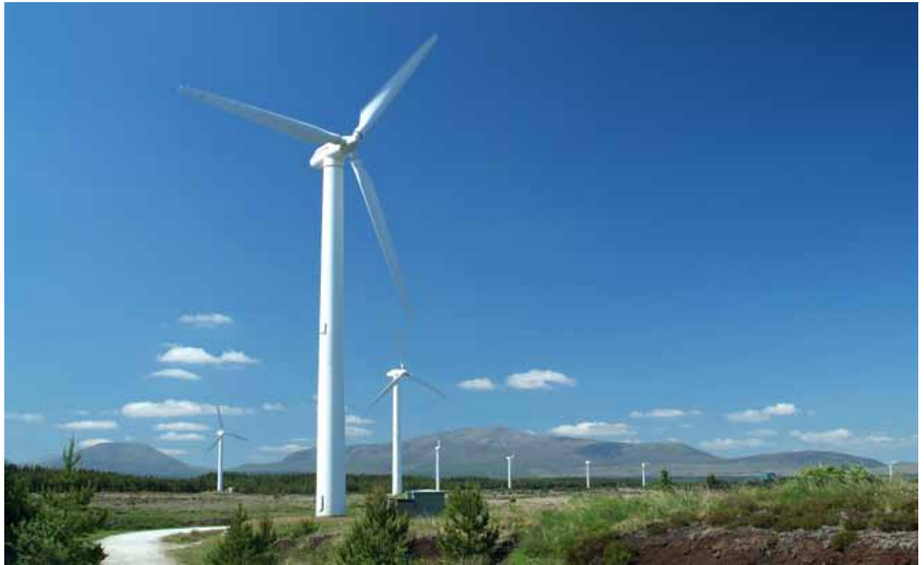
Wind Turbines at Oweninny Wind Farm.
